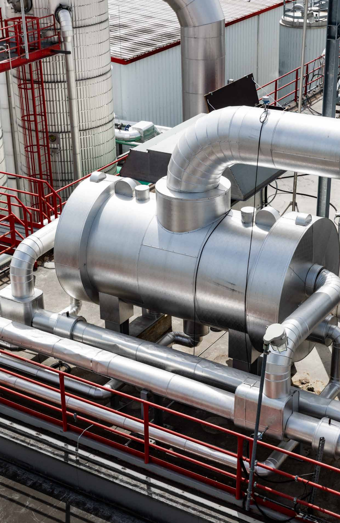
Installed on the roof, the Vahterus steam generator recovers heat energy from ethanol vapour to generate low pressure steam, which is the energy source for Pannonia Bio's stillage evaporation system.
